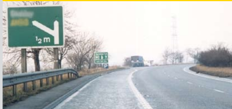
Poor design a lay-by sited before a junction but after an exit sign
